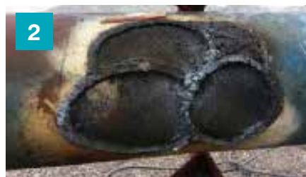
Remove lacing member ends adjacent to the main chord, repair surface of main chord to pass 100% UT inspection
